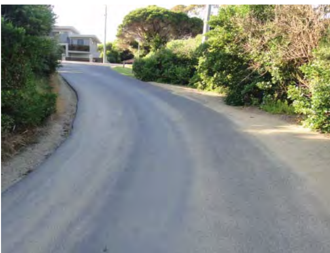
The existing road to the eastern carpark is narrow with no defined pedestrian path. On busy days cars park on the road edges, forcing pedestrians into the middle and making it difficult for cars to pass. Potential to improve pedestrian access and prevent erosion to edges.
