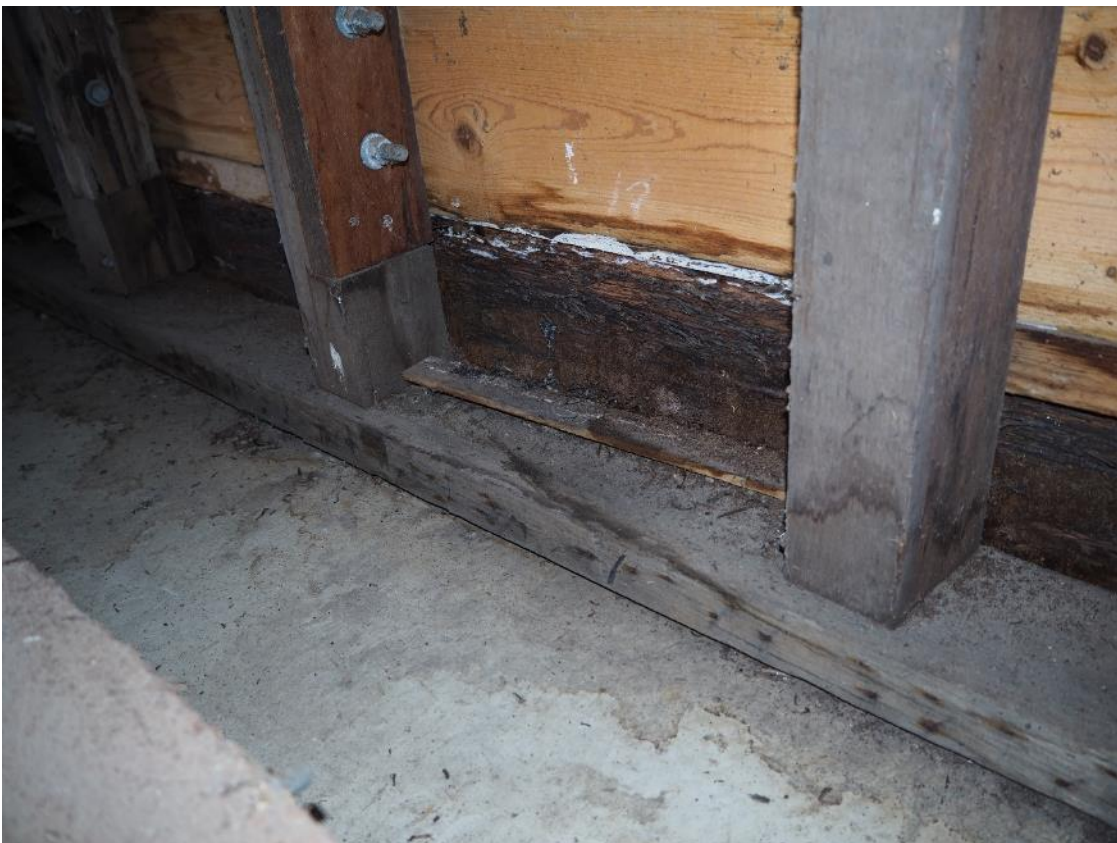
Figure 82: Damaged timber on inside of plinths
