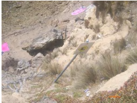
Observation 5 – View of beware unstable cliff hazard sign that has succumbed to the eroding cliff face.
