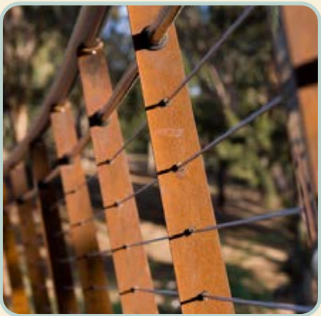
Balustrade in stainless steel and weathering steel
